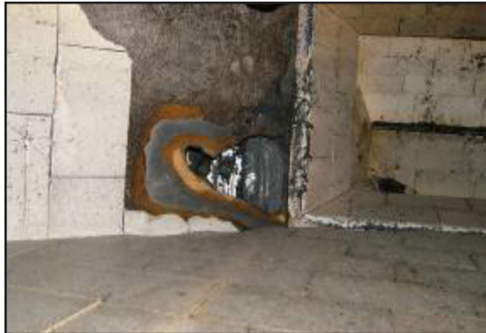
Failure of tile lined chute after 4 months prior to patch weld
